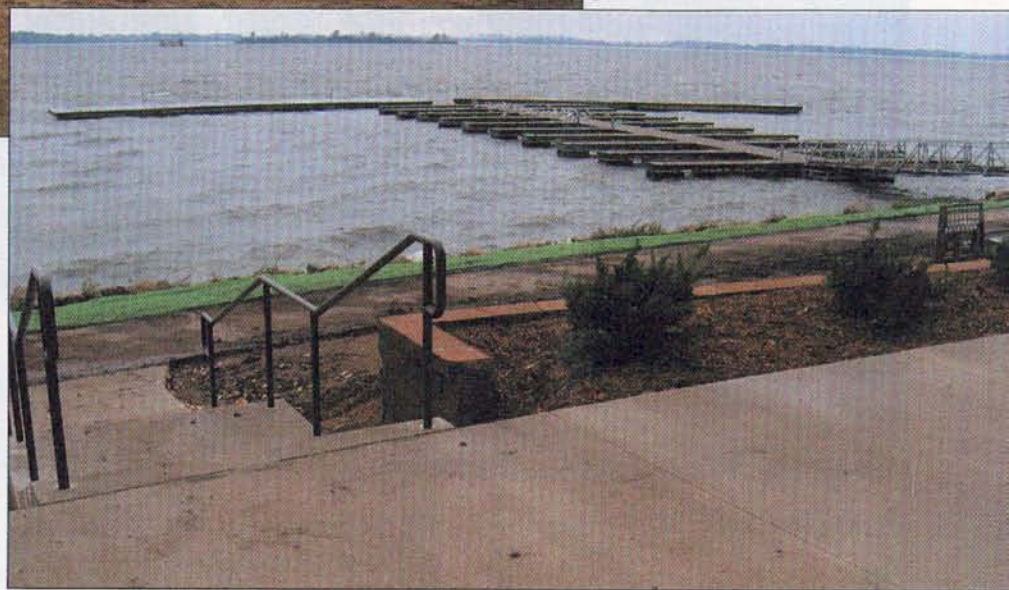
Below: A newly-installed Rixö Model 850 wave attenuator helps pave the way for a new marina in Charlottetown, Prince Edward Island.
